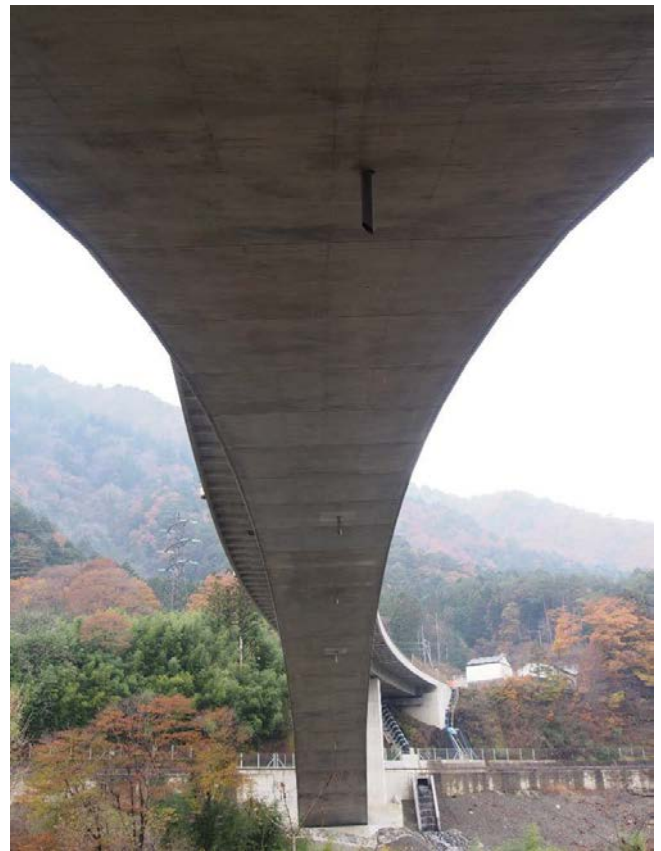
Figure 14. Deviation of arche and curved girder.
