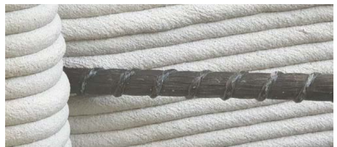
Figure 5. The incorporation of FRP reinforcement into 3D concrete printed cylindrical shell element (Lab. of Construction Materials and Technologies, BME, Budapest) (Photo GL Balázs).
