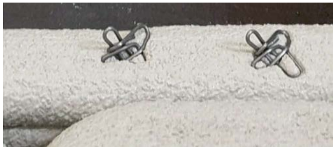
Figure 6. Increase of interlaminar shear in 3D printed concrete by STAREX elements (Lab. of Construction Materials and Technologies, BME, Budapest) (Photo GL Balázs).
