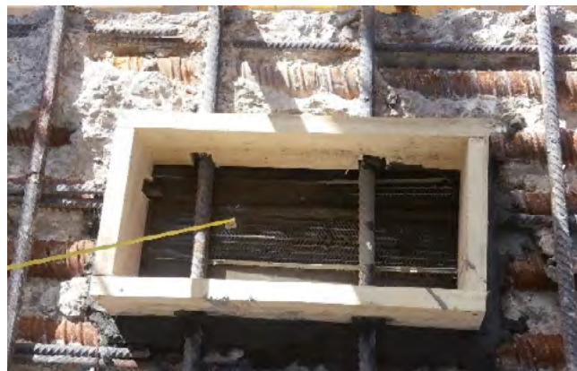
Figure 26. Deteriorated sheath sealing boxes.
