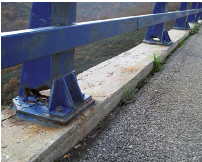
Figure 4. Detail of deterioration in parapets.
