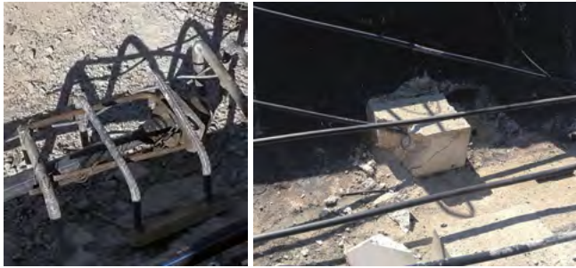
Figure 26. Existing reinforcement in the shell passive anchor block and anchorage failure.
