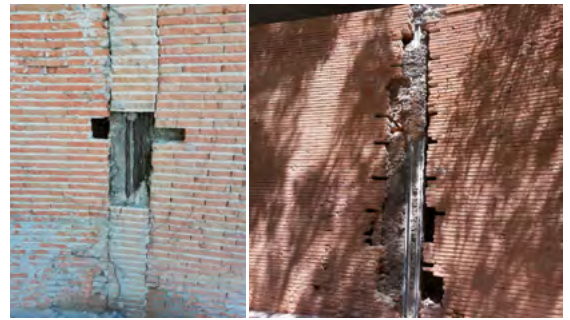
Figure 49. Embedded concrete stiffener and spalled bricks due to corrosion.
