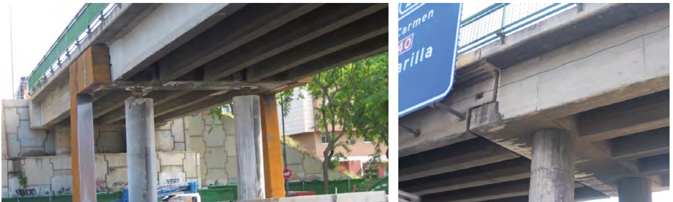
Figure 13. Overpass in the A-30 highway in Murcia. Span enlargement solution with half-lap joint in the deck.
