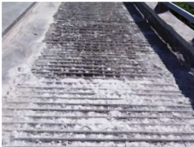
Figure 22. Existing reinforcement exposed.
