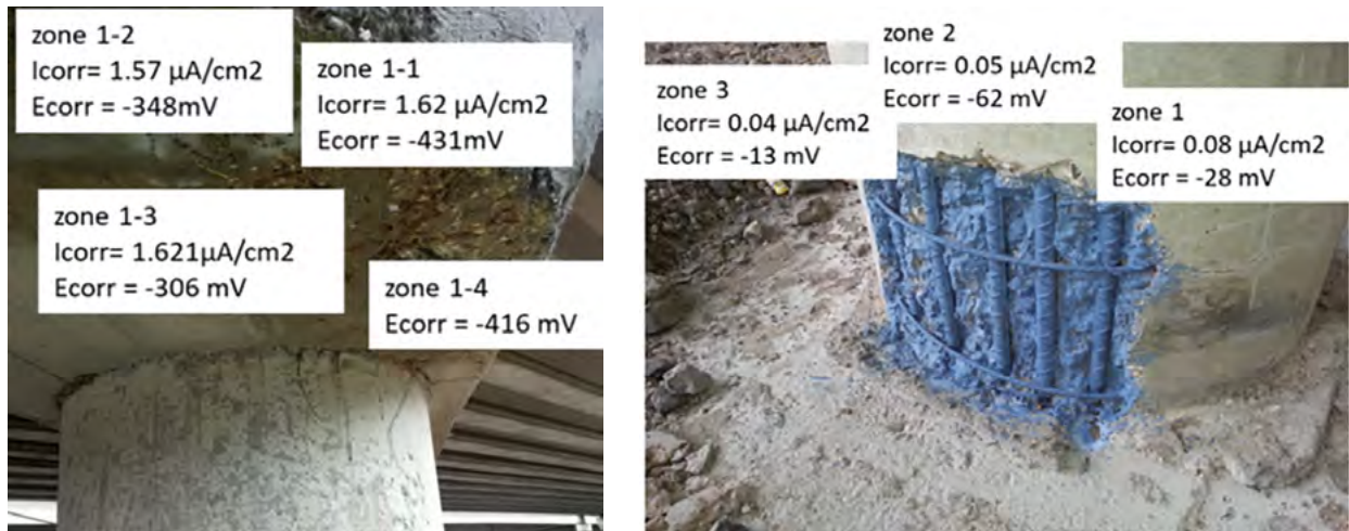
Figure 16. Left: corrosion values on the viaduct pier cap prior to repair; right: corrosion values during repair on a viaduct pier.
