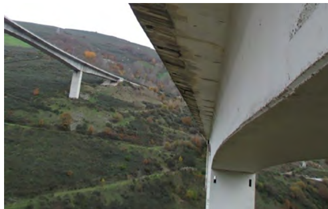
Figure 8. View of the state of the right edge of the existing extended deck.
