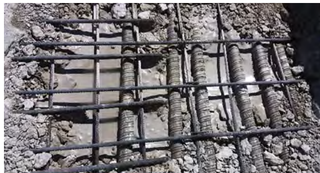
Figure 25. Post-tensioned sheath details with deterioration.
