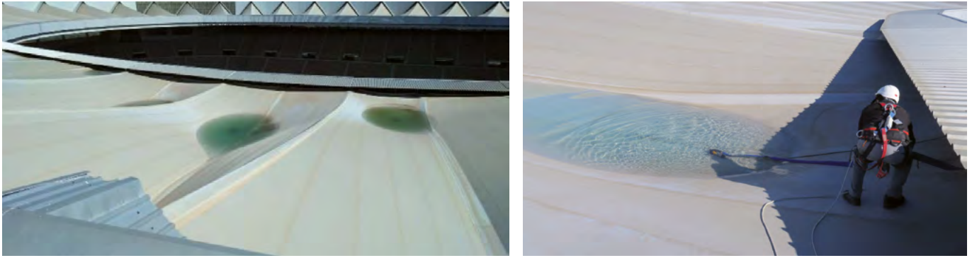
Figure 5. Ponding on the roof. Credit: schlaich bergemann partner
