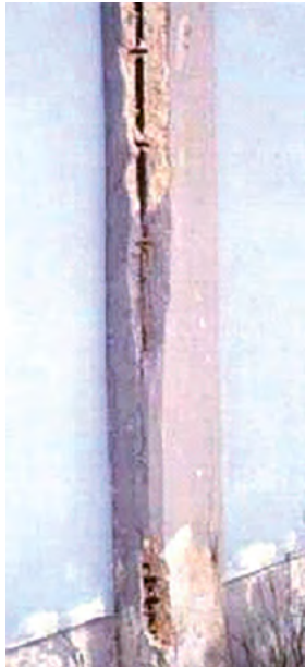
Column with corrosion stains at different heights
