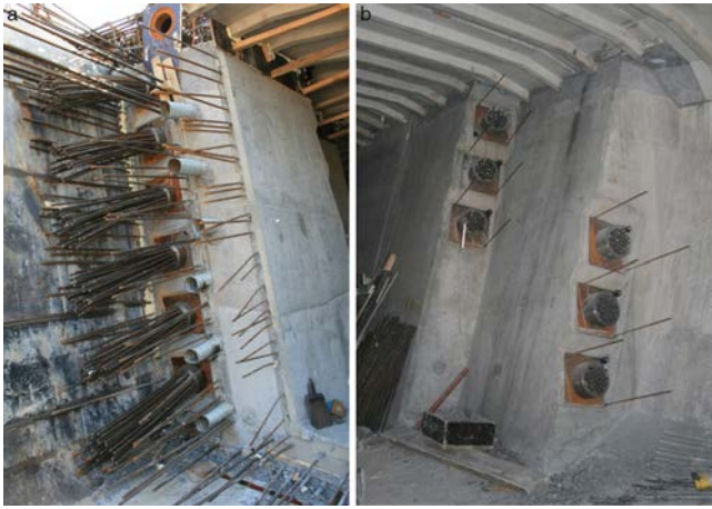
Figure 28. Continuity tendon anchorages and crosslinked wires and active anchorages at cantilever front; passive steel anchorages.
