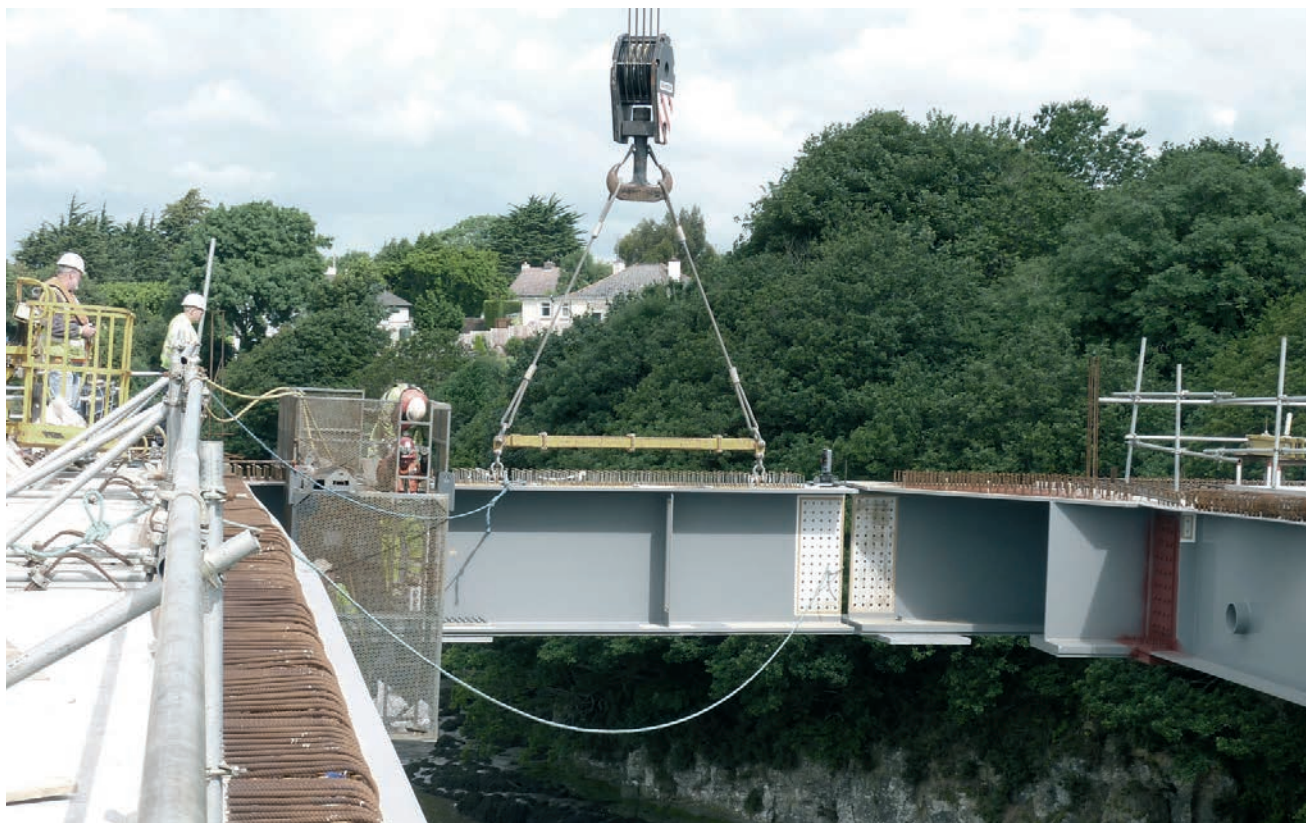
Figura 40. Colocación del tramo de cierre del vano. Figure 40. Installation of the closing segment of the span.
