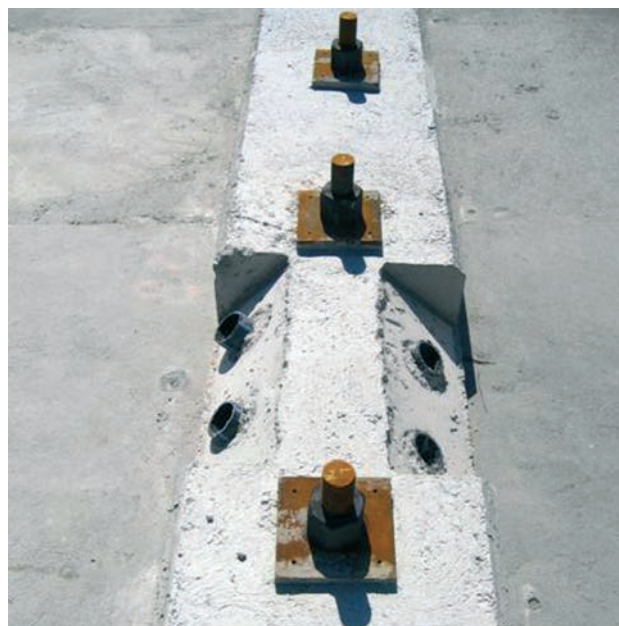
Figura 17. Tacón de anclaje de barras verticales y diagonales File 17. Anchor of the vertical and inclined bars
