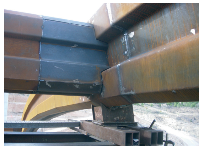
Figura 40. Riostra entre arcos, péndola y apoyo cimbra Figure 40. Inter-arch brace, hanger and falsework support
