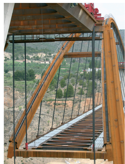
Figure 21. Riostra de bowstring Figure 21. Bowstring brace
