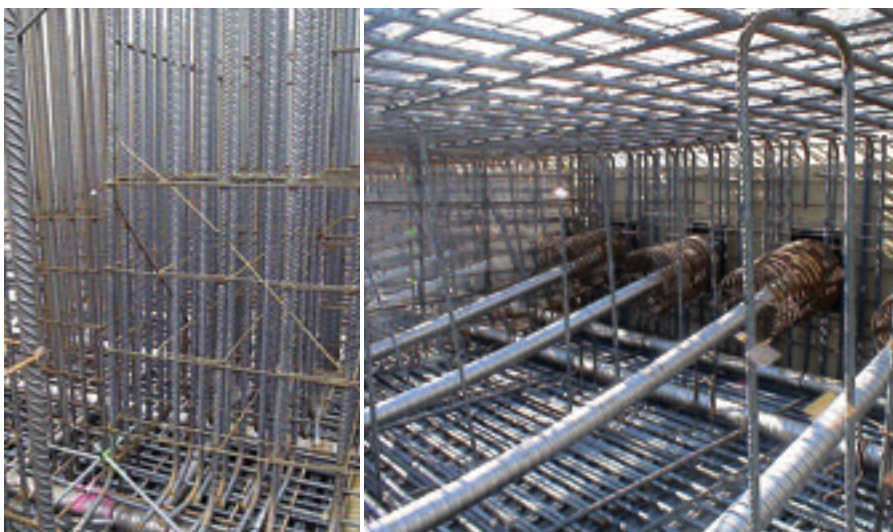
Figura 3. Detalle de arranque de núcleo central y fijación de cabezas al encofrado. Figure 3. Detail of the foot of the central core and attachment of the prestressing heads to the formwork.
