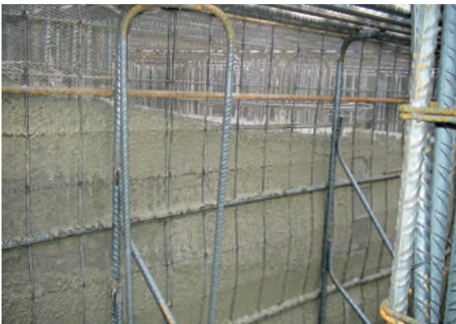
Figura 5. Detalle de junta vertical con nervometal. Figure 5. Detail of vertical joint with nervometal (metallic reinforcement).
