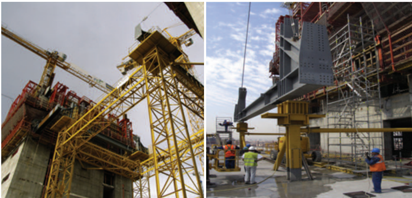
Figura 22. Apesos de cerchas en planta PT1 (izda.) y en PT 2 y PT3 (dcha.). Figure 22. Supports for PT1 (left) and PT2 and PT3 (right) trusses.
