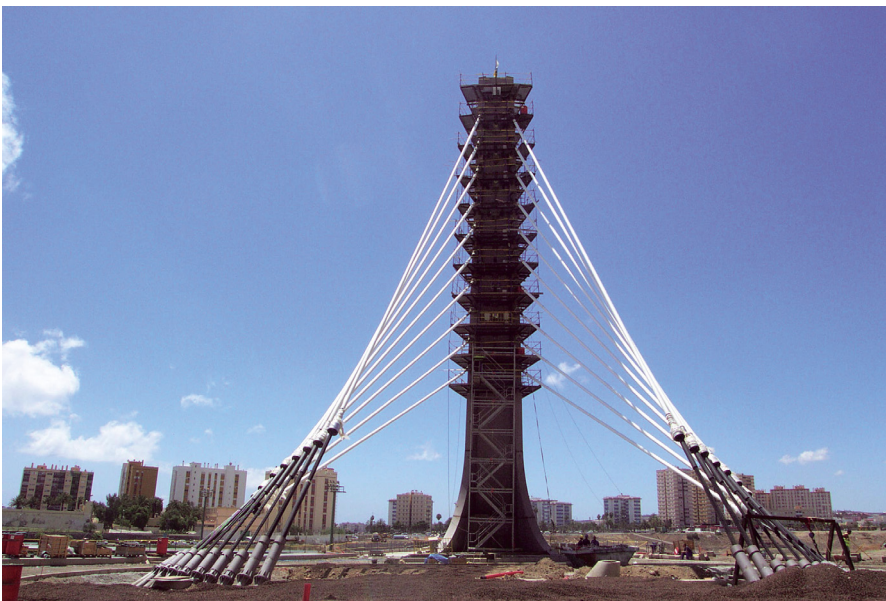
Figura 37. Vista trasera de los tirantes durante el montaje. Figure 37. Rear view of the stays during assembly.
