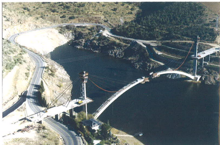
Foto 3. Vistas del arco durante procedimiento constructivo. Picture 3 Views of the arch during the construction procedure.
