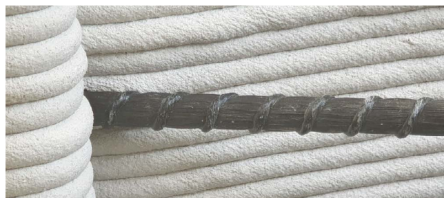
Figure 5. The incorporation of FRP reinforcement into 3D concrete printed cylindrical shell element (Lab. of Construction Materials and Technologies, BME, Budapest) (Photo GL Balázs).
