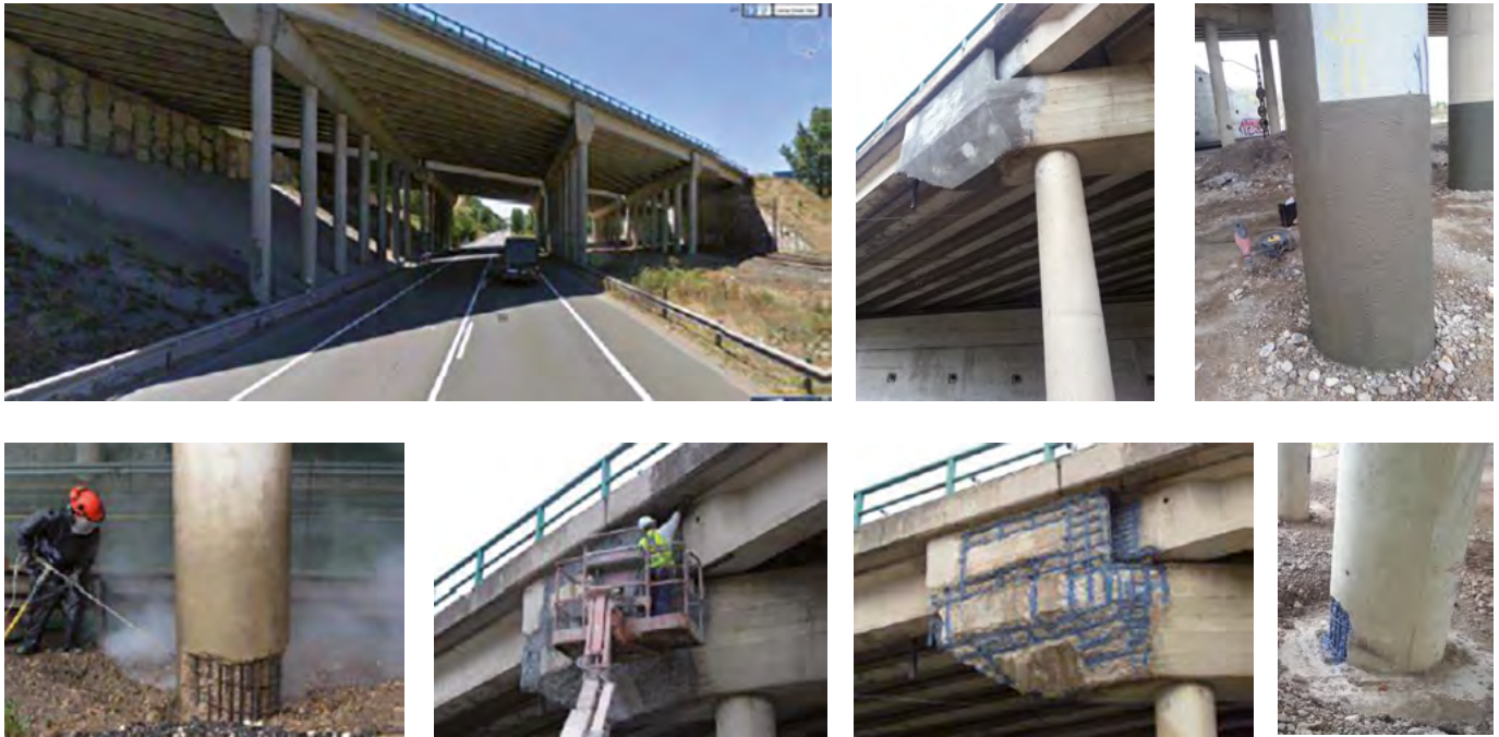
Figure 5. Viaduct on motorway AP-I (Spain) patch-repaired. 3
